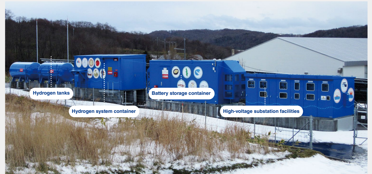
An entire landscape of the microgrid facilities in Atsuta, Ishikari City (photograph taken in December 2021)
