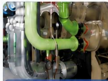
CHILLED WATER SYSTEM
