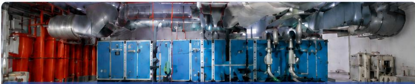
AIR HANDLING UNIT (AHU)
