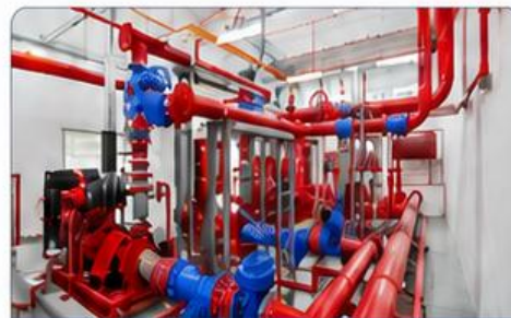
FIRE PUMP ROOM
