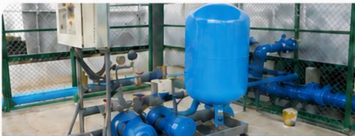
CITY WATER PUMP
