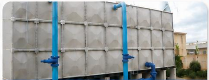
DOMESTIC WATER TANK
