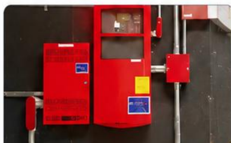
FIRE ALARM SYSTEM
