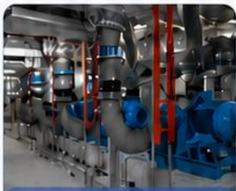
HVAC WATER PUMP SYSTEM
